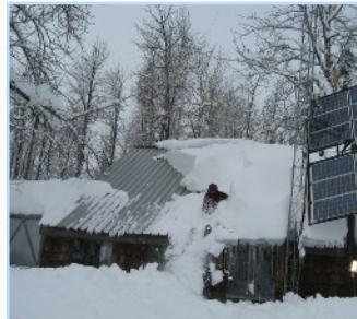
Snow avalanching off Yentna Station roof.
